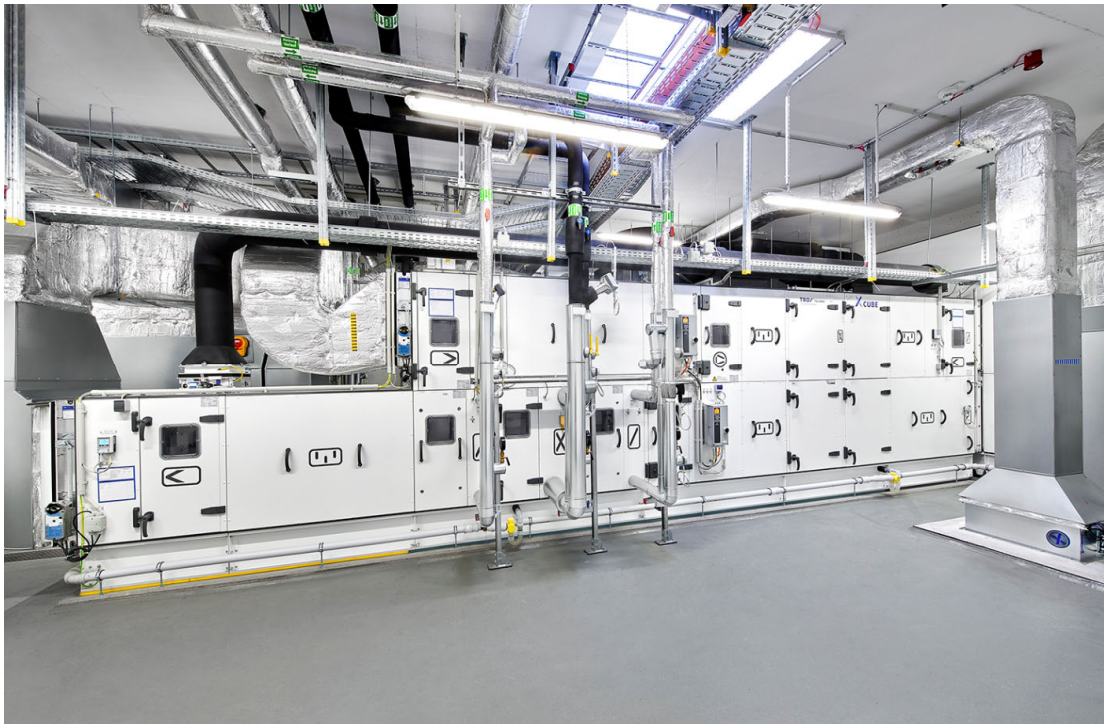
@TROX: Combined supply and exhaust equipment of the X-CUBE series (one of 51 X-CUBEs)
