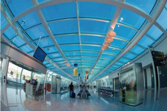
Brazil: TROX swirl diffusers distribute fresh air to the halls and corridors of Rio de Janeiro's Santos Dumont Airport.
